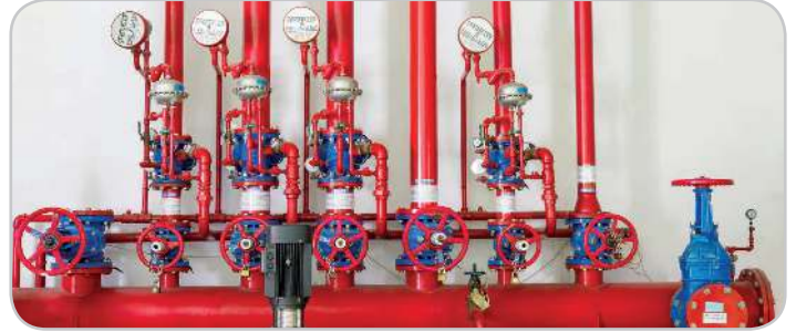
The weekly, quarterly and annual flow testing of fire sprinkler systems is one of the many areas we can assist you
